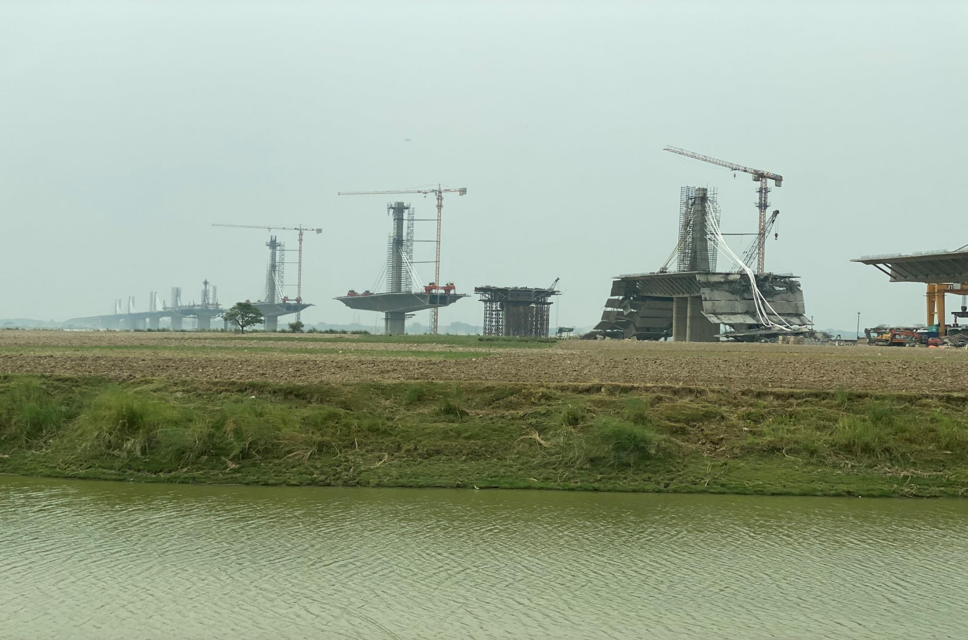
Sultanganj Bridge Collapse of Cantilevers 2022-04
